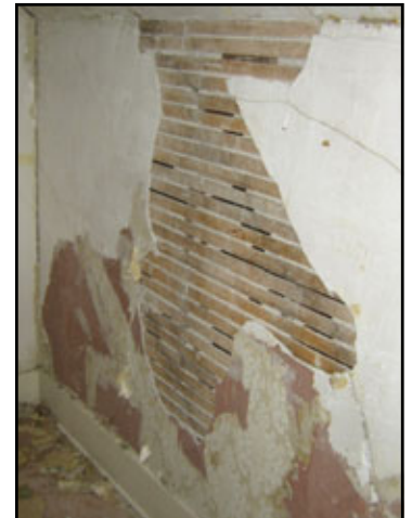
Extensive wall damage was revealed under layers of paint & wallpaper.
